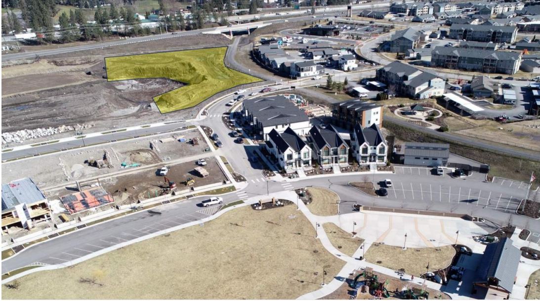
Photo depicting remaining area of Phase 3 site that is currently being worked to determine level of non-structural fill material.
