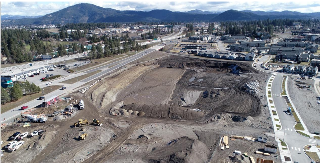
Photo showing site embankment work on the north side of the Phase 3 site.
