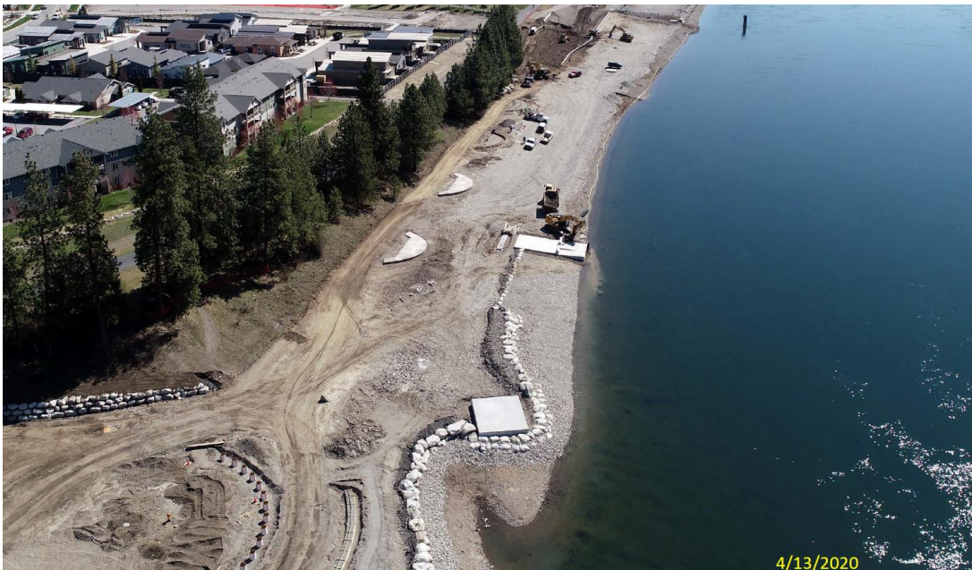
Project Site: Closeup View of Beach Area, Dog Water Park Area & Water Access Pads (concrete pads usable for water access at summer water levels)
