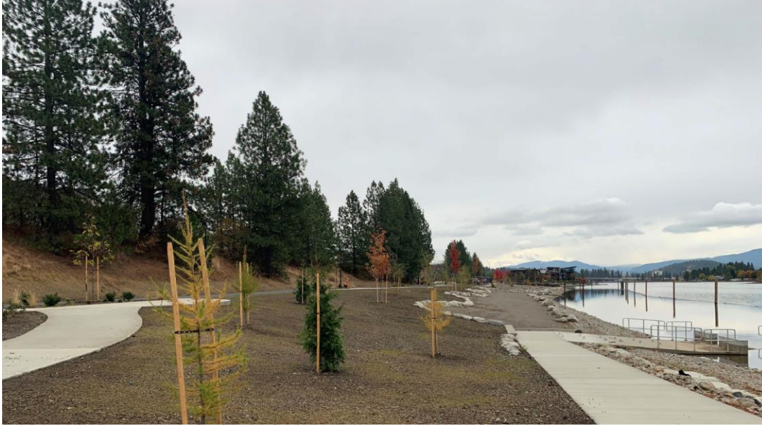
Project Site: Showing concrete flatwork and landscaping located along the river's edge.
